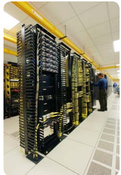
Figure 1. Equipment and Cable Racks
