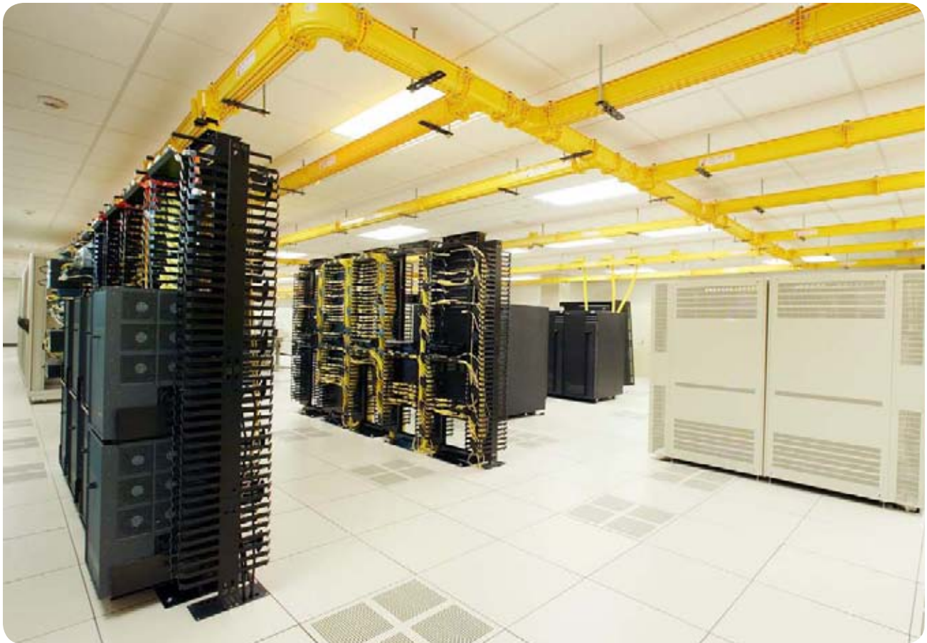
Figure 3. Data Center with Flexible White Space
