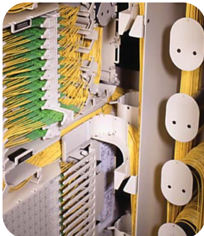
Clearly defined cable routing paths
