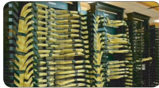
Figure 6. ADC KRONE Glide Cable Management System
