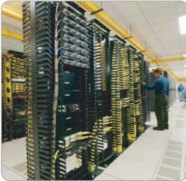
Figure 1. Equipment and Cable Racks
